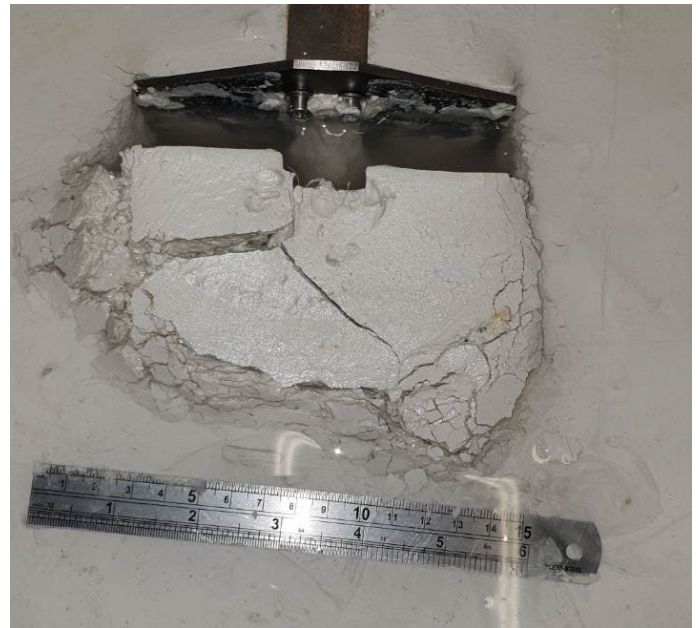
Figure 9 Gapping behind plate
